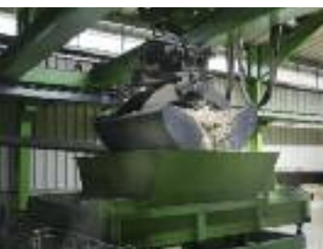
The feeding of the reactor occurs depending on the level through the vibration groove and the lock lid.
